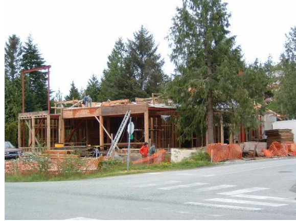
The Cedar Corners commercial development in Tofino will be the first gold LEED restaurant in North America
